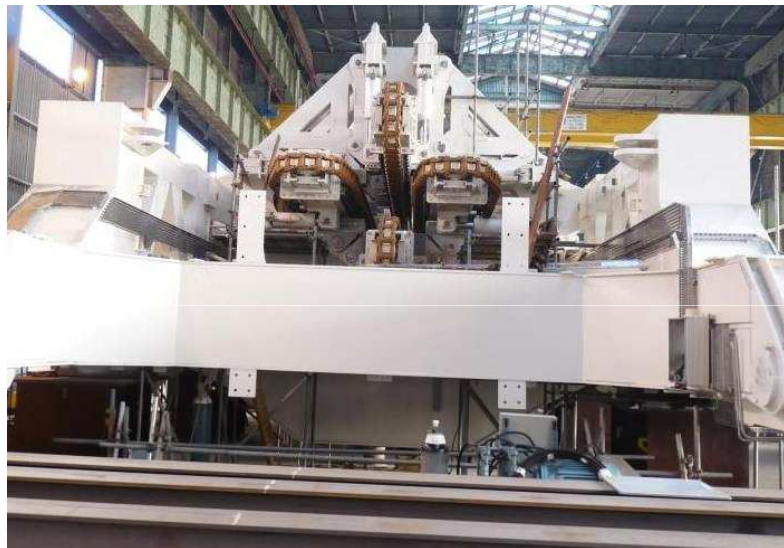
4 Track 150Te Tensioner under construction as part of a vertical tower lay system. The Tensioner is constructed in sub-assemblies and then brought together as a unit within the tower.
