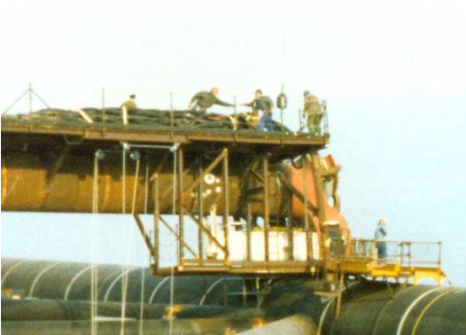
Pin Release System mounted from Jacket Lifting Beam.
