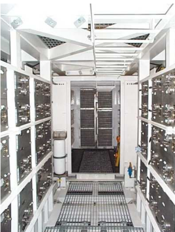
Walk-in view of typical Upending Control Centre
