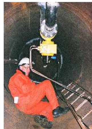
Commissioning Vent Valves within Jacket Legs
